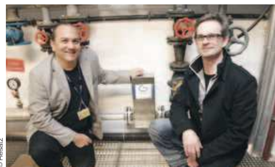
: GRANDER at the airport (l to r): Karl Heinz Santruschitz, head of in-house technical staff and Robert Strobl, building project representative OIB
